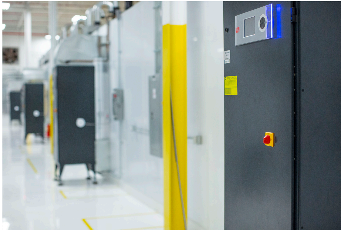
STULZ Air Conditioners in Denver, CO (photo courtesy of Medicine Man Technologies)
